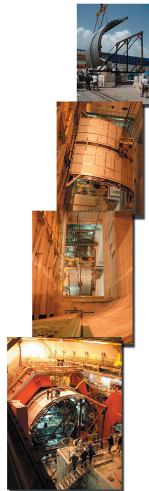
The 25-ton support structure for the EMCal was lowered 50 feet to the ALICE experimental cavern and installed in November, 2007.
