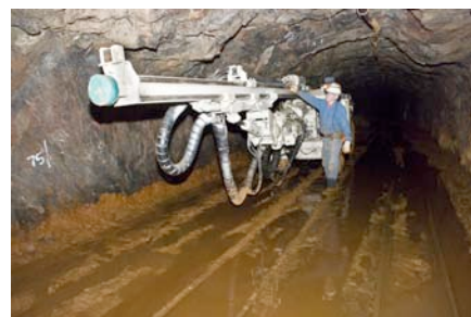
Figure 11: Sanford Lab Underground Operations Foreman Jack Stratton behind the 20-foot boom of the Jumbo drill on the 4850 Level
