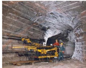
Figure 2: Example of results of well-executed controlled blasting. Photo taken on 240-m level of Atomic Energy of Canada Underground Research Laboratory at Pinawa, Manitoba. Lack of blast damage and minimal use of rock support evident in this photograph.
