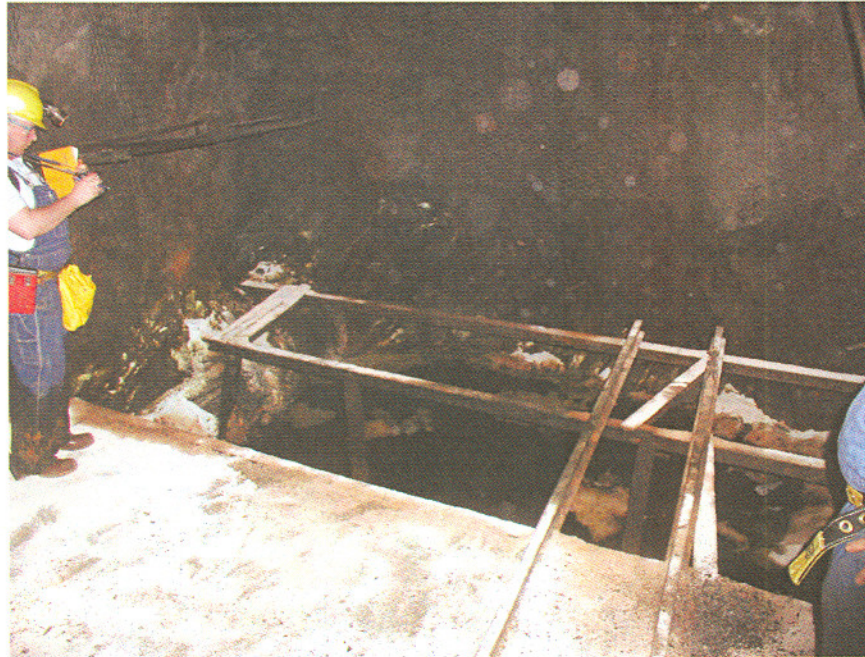
Photo 9. 3800 Level Fuel Storage area. Note Spill Shark absorbent has been liberally applied.
