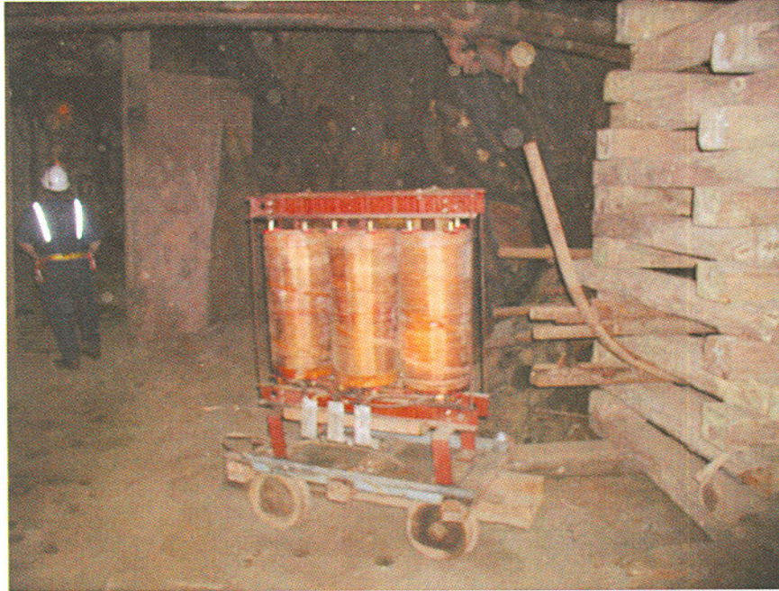
Photo 6. 1700 Level, 7 Ledge shop area, dry core transformer abandoned in place. Note cribbing for roof support.
